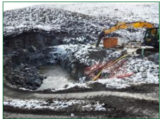
Pictured: Final intake rock trimming at Abhainn Gleann Nam Fiadh before works continue
